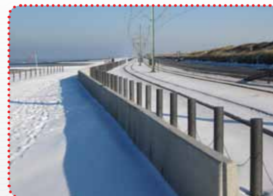
In the fight against sand, a pilot project got underway in October 2012 in which De Lijn is a partner. Alongside the Kustbaan (Coastal Road) between Middelkerke and Oostende, a 330-yard length retaining wall was put in place with high concrete edging slabs.
