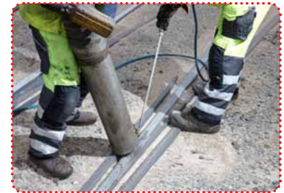
A sand "hoover" is used to clear the tracks from sand and leaves. The build-up of sand may cause the tram to get stuck or even get derailed. Leaves act to make the tracks more slippery, which in turn makes for a longer stopping distance.
